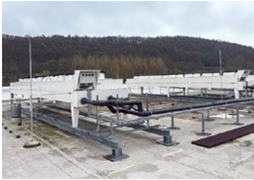
Ambient air cooler installation on the roof of the GF Piping Systems plant in Dautphetal (Germany).
